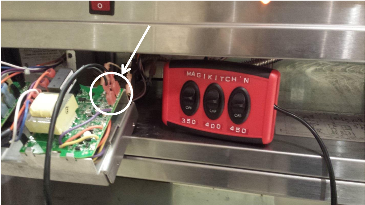
Figure 9: Unplug the T-Stat wires from the first controller and replace it with the leads from the Calibration test tool, as shown above (leads do not have to be in any certain order/position).
